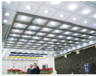
LED 照明設備
